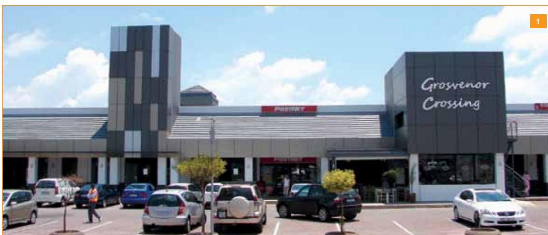
1 As part of the upgrade, a new aluminium panel façade has been installed above the malls.
